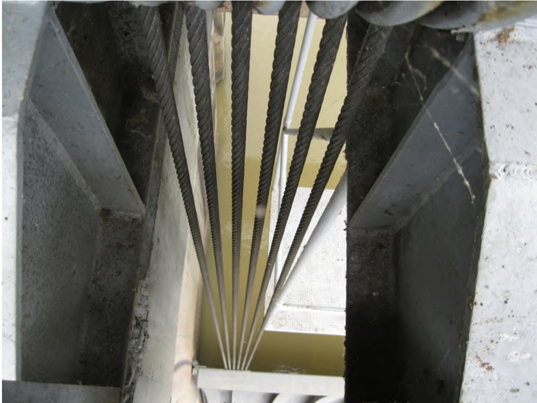
Figure 16-4. Wire Ropes for Lifting a Tainter Gate.
