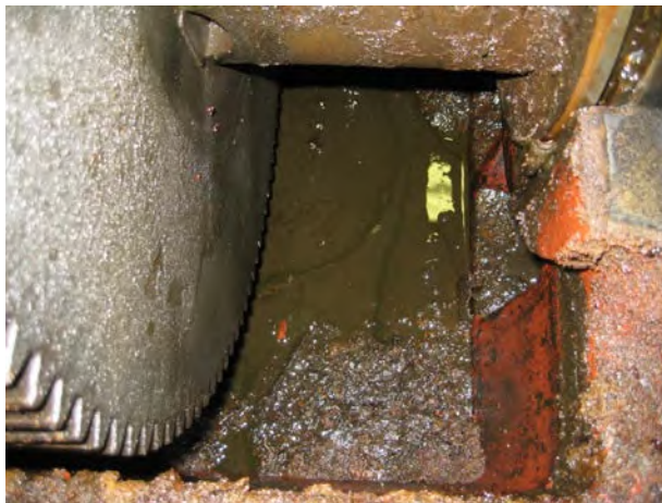
Figure 14-8. Gear Reducer in Need of Cleaning and Flushing.
